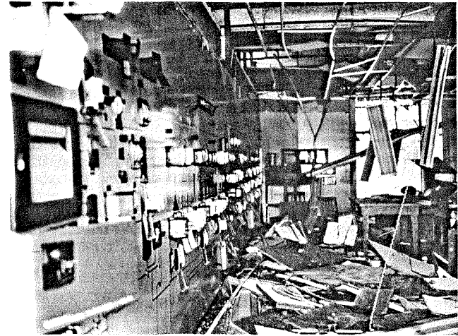
Figure 5. Every instrument in the main control room had been blown out of its case.
